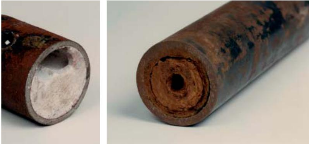
Boiler scale on water side
